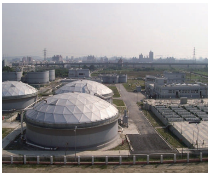
▲ Image 16 / Fengshan River Sewage Treatment Plant and Reclaimed Water Treatment Plant
