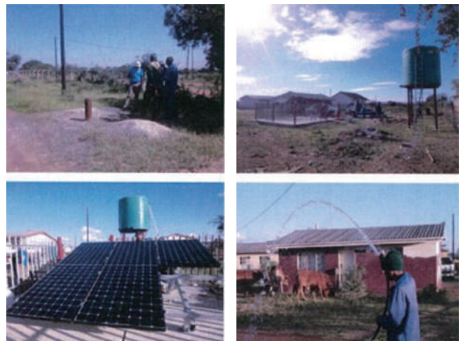
▲ Image 18 / Assisting set up of solar photovoltaic pumping systems in eight middle schools
